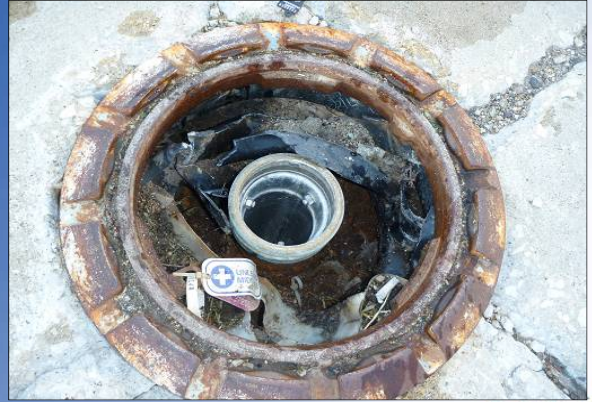
Obviously Compromised Containment...
