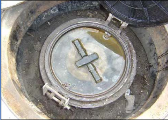
Inadequate Spill Containment
